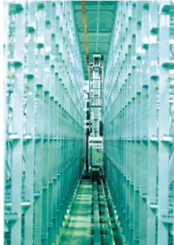
Automatic Warehouse(unit type)
